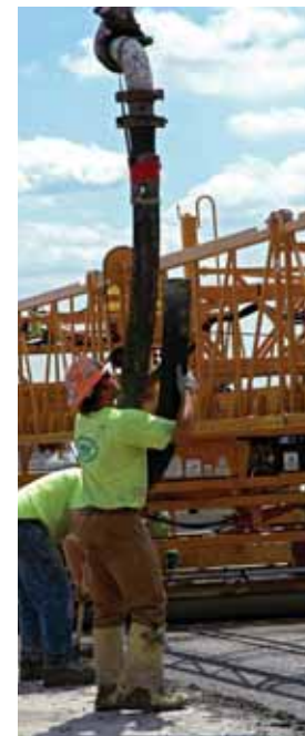
Workers operate concrete pump in the building of the I-94 Business loop of Memorial Bridge in North Dakota. Photo courtesy of Mike Kopp, North Dakota Department of Transportation, 2008.
