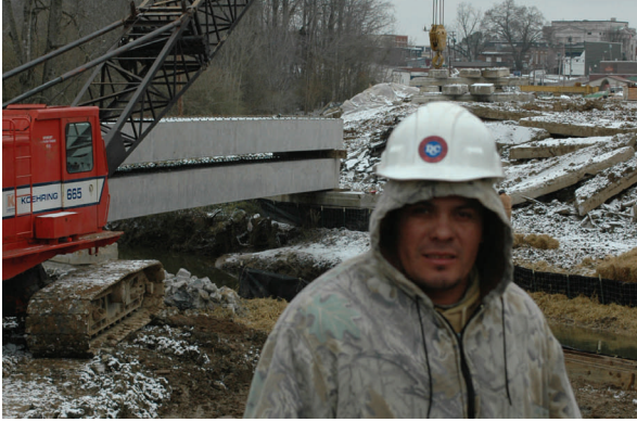
Cesar Gonzales, Laborer Trainee, with Dement Construction on a Bridge Replacement project on State Route 22 in Carroll County.
