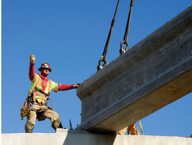
Josh Littleton, Carpenter for Bell & Associates Construction on the I-40/White Bridge Road/Robertson Road/Briley Parkway Phase Two Interchange Modification project in Nashville
